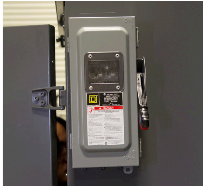
FIGURE 14: TYPICAL FACTORY SUPPLIED DISCONNECT ▼
