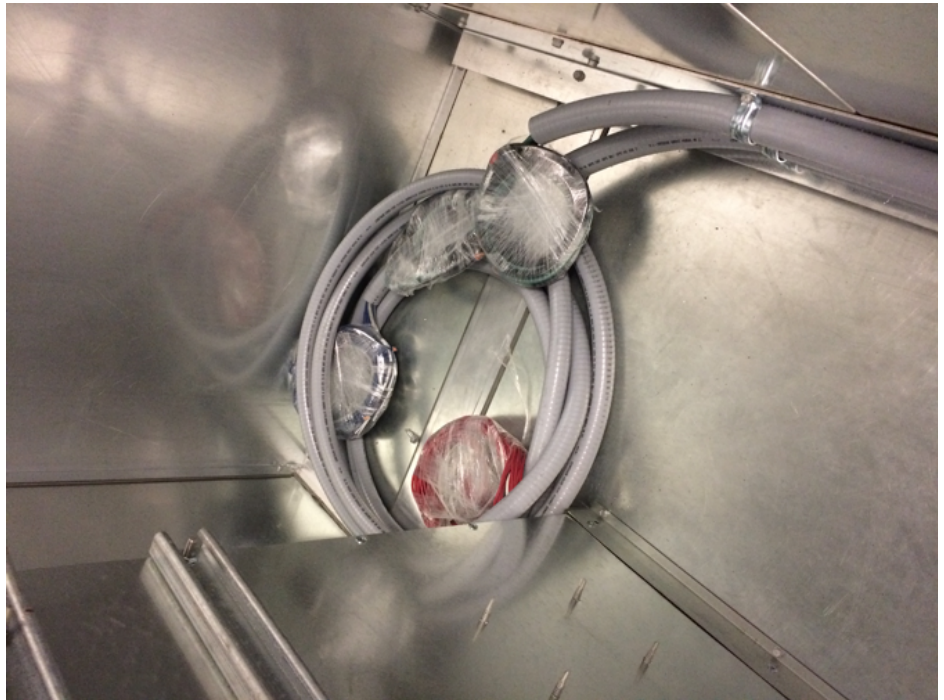
FIGURE 7: HIGH VOLTAGE WIRES SPOOLED ▼
