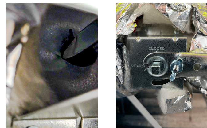
Figure 10 Example installation of inadequate sealing.
